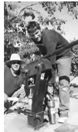
Murwira Orphanage volunteers, Bruce Hamberger (left), and Josh Schaa (right) installing a submersible solar water pump next to an existing hand pump.
